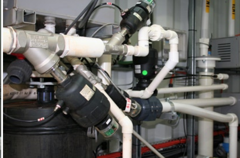
Left: Control panel in the MIEX® Pilot Plant, featuring Bürkert pneumatic valves working in concert with Allen-Bradley IO. to control processes within the plant. Right: Feature of Bürkert process valves with integrated position feedback.
